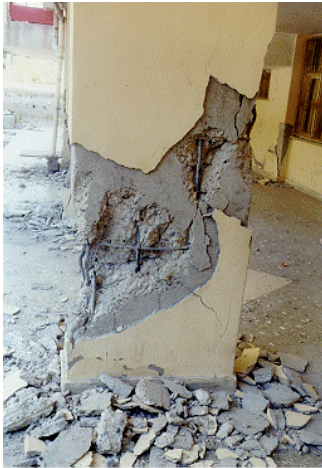
Column shear failure
